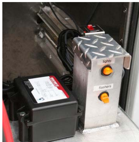
An onboard battery powers cabinet lights and the trailer's emergency flashers when the generator is not running. Helpful for dark nights.
