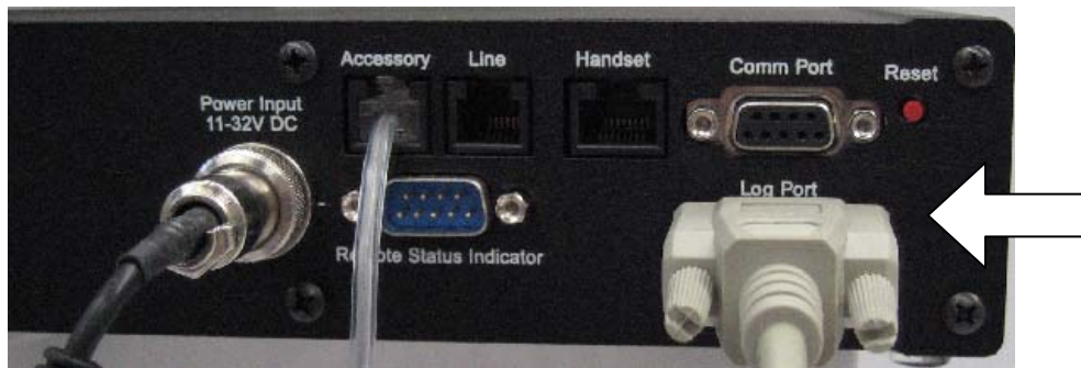
Figure: Serial cable connected to Log Port
